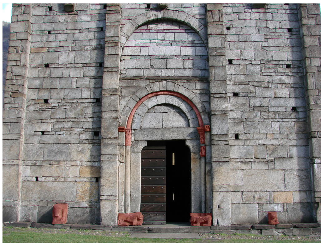
Figure 1. Lower part of western facade with main entrance of the San Nicolao church in Giornico. The soapstones are marked with red colour.
